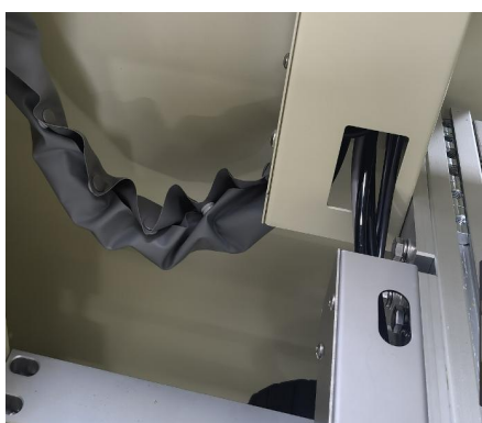
Protection for all connecting wire
